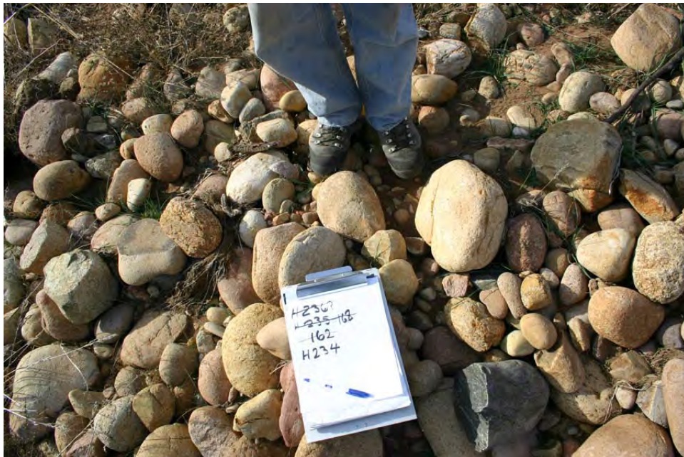
Plant (234) – Missing, scour.
