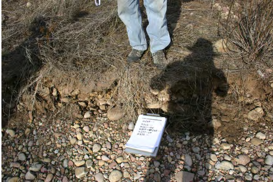
Plant (256) – Missing, bank erosion.
