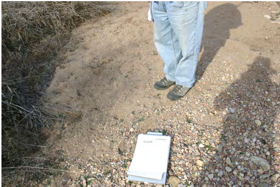
Plant (265) – Missing, scour.
