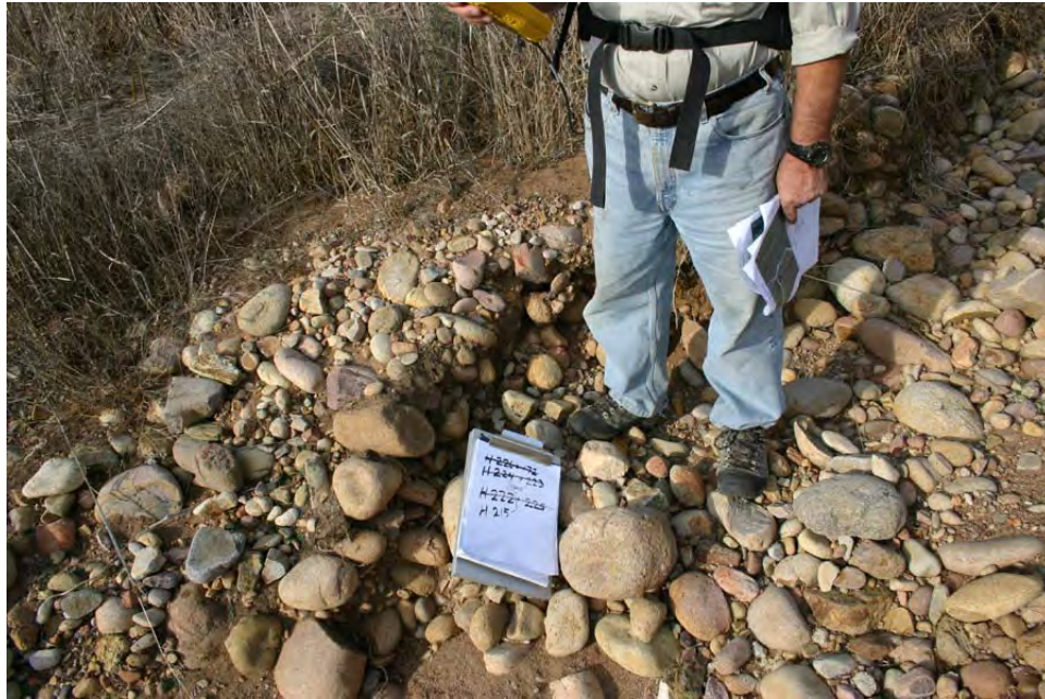
Plant (215)- Missing, scour or bank erosion.
