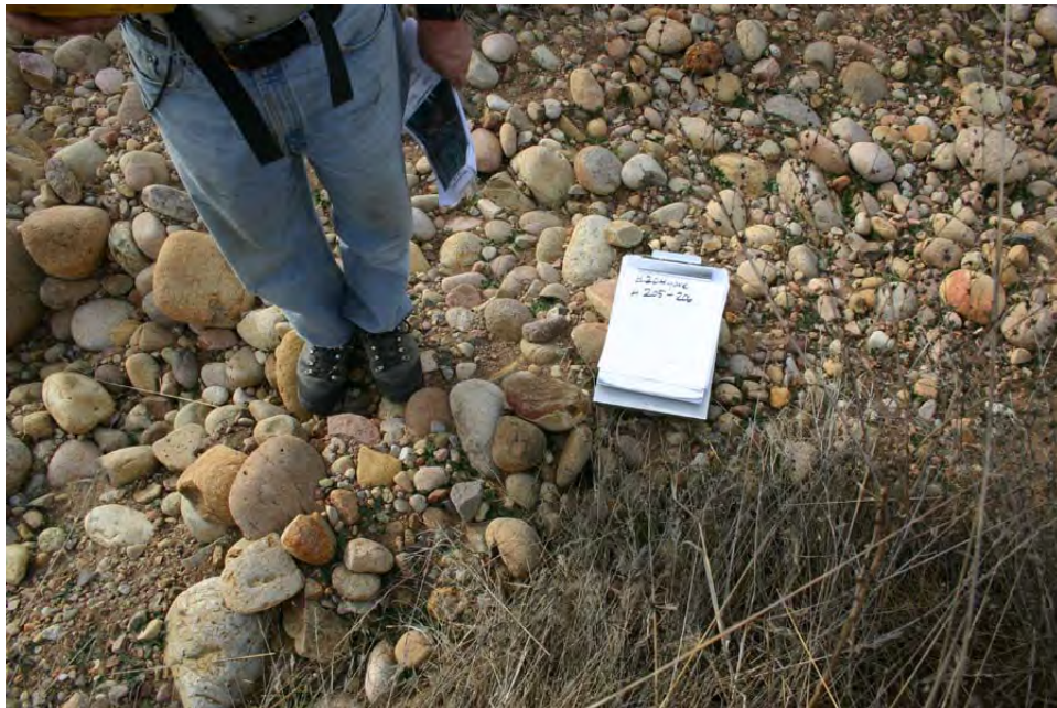
Plants (205 & 206) – Missing, scour.
